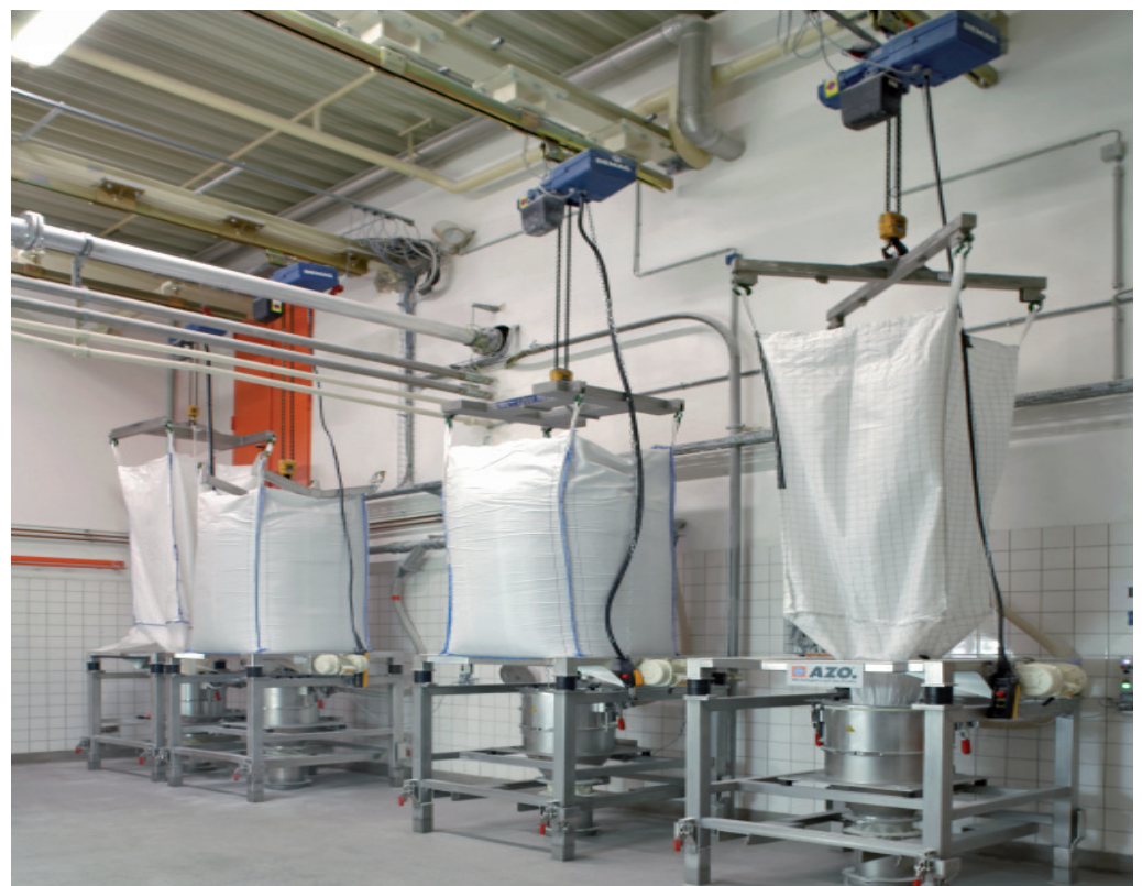
Figure 19: FIBC emptying (Source: AZO® GmbH + Co. KG)
